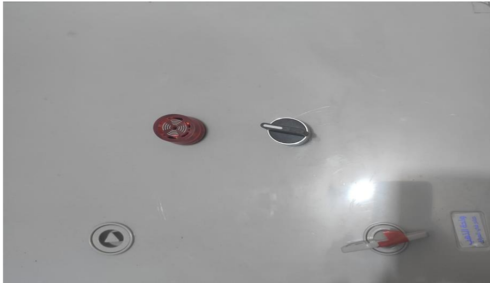
Figure (3.2): The Electric Switch and also The Electric Buzzer
