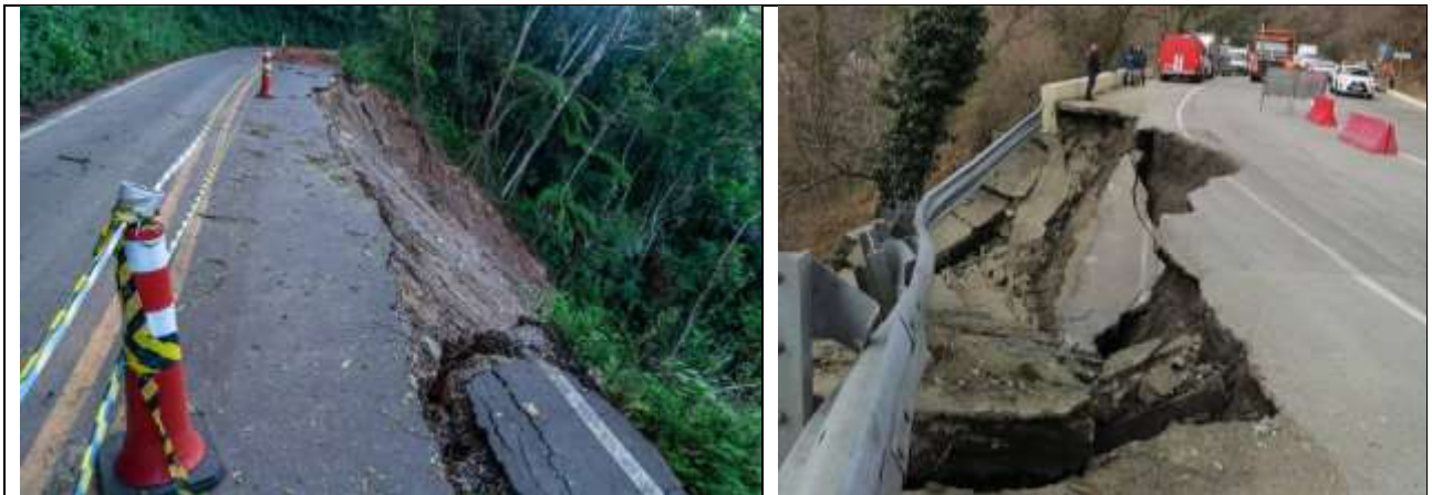
Figure 2. Landslides of the slopes of the embankment of the road.
